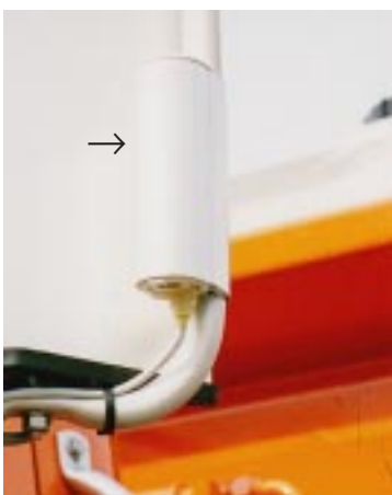
air/pavement temperature sensor Sprague Company Canby, Oregon
