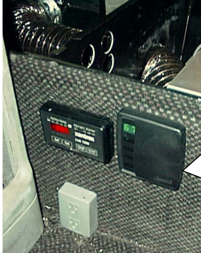
Amp hour counter and Air conditioner control & receptacle
