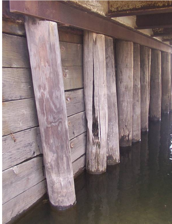
Figure 1. Timber pile deterioration
