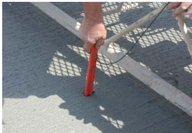
Figure 3. Digital data logger placement
