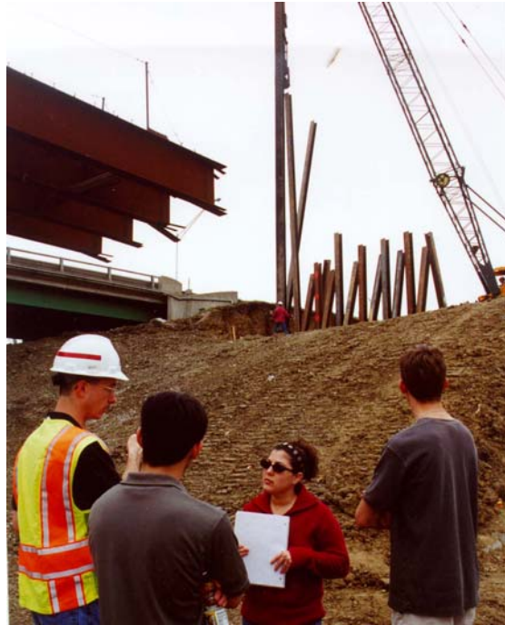
FIGURE 2. Students Visited a Construction Site on the Interstate 235 Project in Des Moines, Iowa
