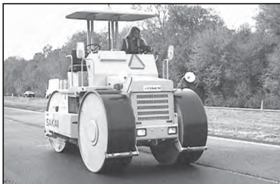
A consistent roller pattern helps achieve density, an important quality for hot mix asphalt longevity. Photo courtesy of the National Center for Asphalt Technology.
