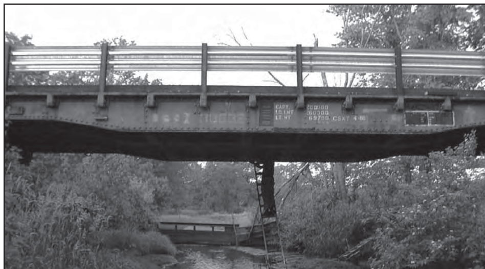
With careful design, engineering, and analysis, Buchanan County is experiencing success with cost-effective railroad flatcar bridges
