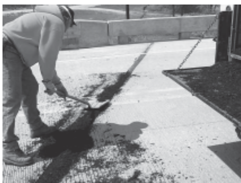
Rubber particles are spread and then sealed into the expansion joint. Photo courtesy of the Iowa DOT.
