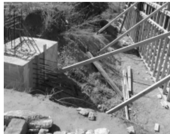
The area excavated to install concrete abutments during bridge construction must later be backfilled. Photo provided courtesy of Iowa DOT District 6.
