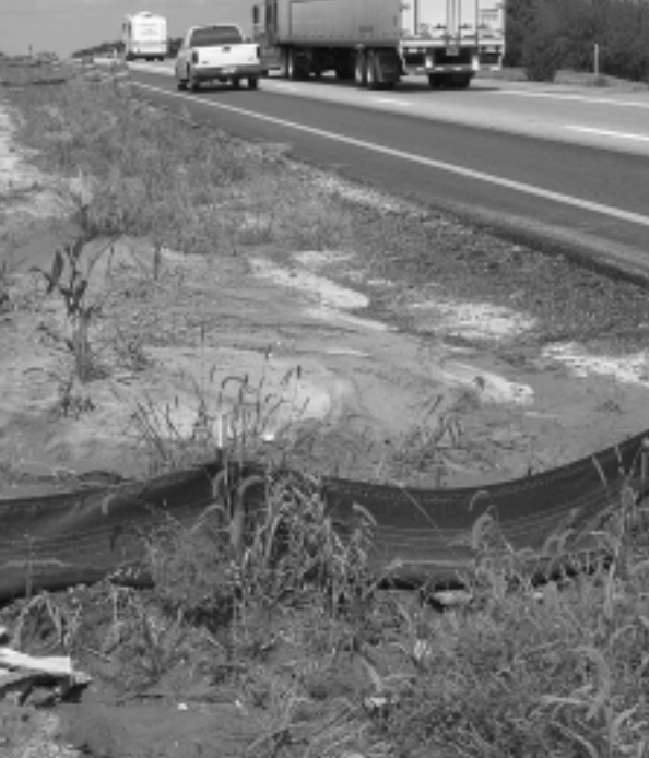
A silt fence is placed near a slope drain to prevent soil and silt from washing down the right of way.
