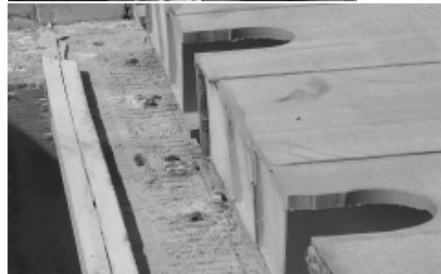
Top: Span 2's concrete deck is reinforced by a mat of FRP. Bottom: Span 3's FRP deck is placed.
