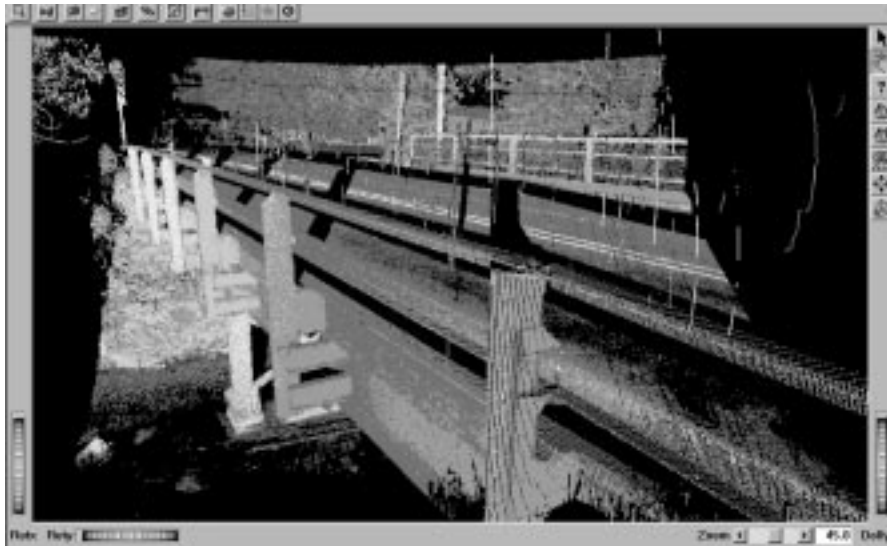
Laser scanned 3D images of existing bridges, like this one in Pennsylvania, could help agencies reduce rehabilitation costs.
