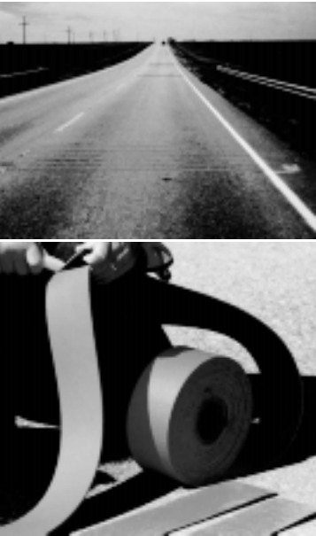
Removable orange rumble strips warn drivers approaching a work zone. Photos courtesy of Eric Meyer, University of Kansas, and Advance Traffic Markings.
