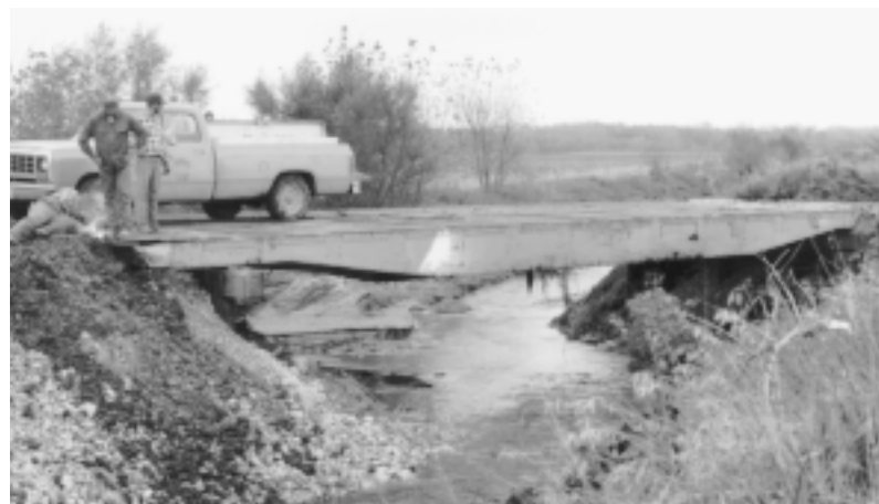
Construction of the Tama County RRFC bridge. Photo courtesy of the Tama County engineer's office.
