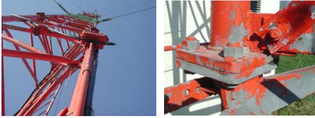
Figure 11. Details of Ashland central mast. Significant paint flaking is observed but minimal loss of galvanization.
