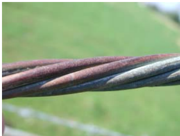
Figure 9. Detail of Ashland guy cable showing minimal corrosion.
