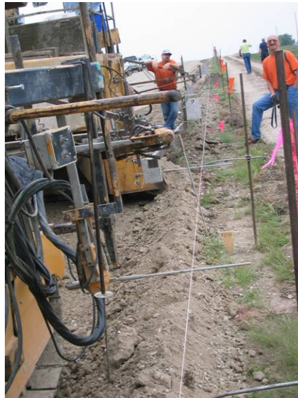
Figure 1. Sensors Used to Read String Lines
