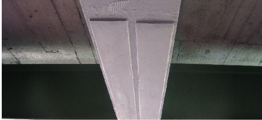
(a) Beam 4 in the east end span
