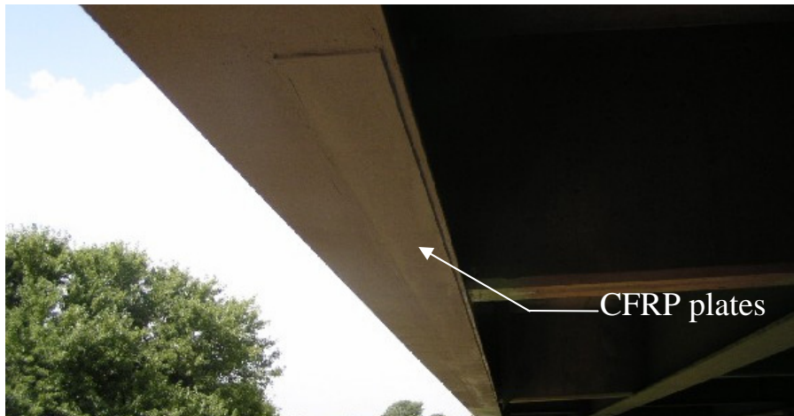
(c) Bottom of bottom flange of Beam 6 in the east end span
