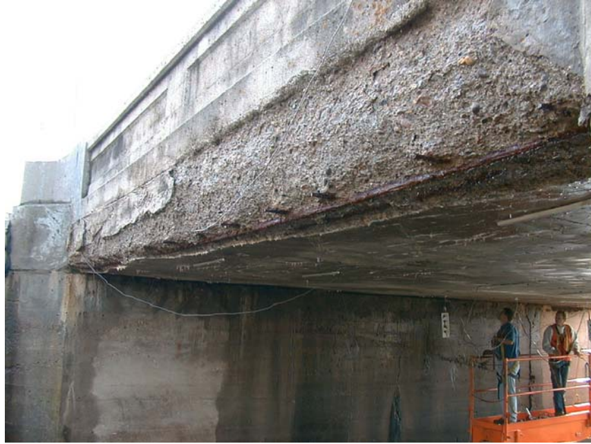
FIGURE 1 Corrosion of Reinforcing Steel and the Corresponding Deck Concrete Deterioration.
