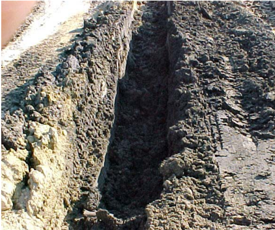
FIGURE 2 Severe Rutting Due to Construction Traffic
