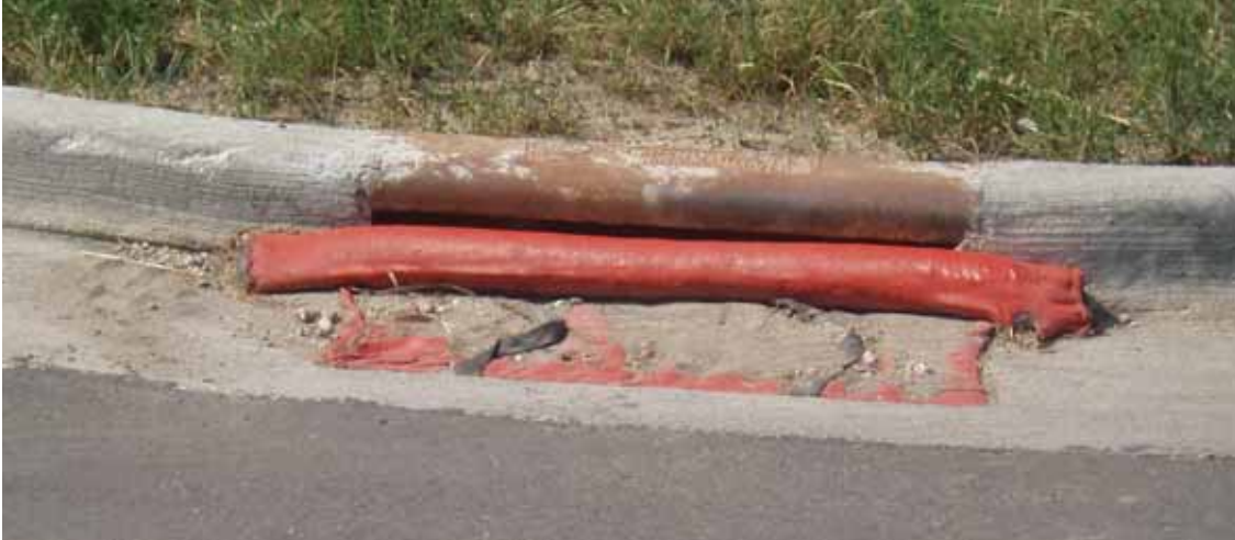
Figure 3.16. Inlet sediment control (Source: Department of Civil, Construction, and Environmental Engineering, Iowa State University)
