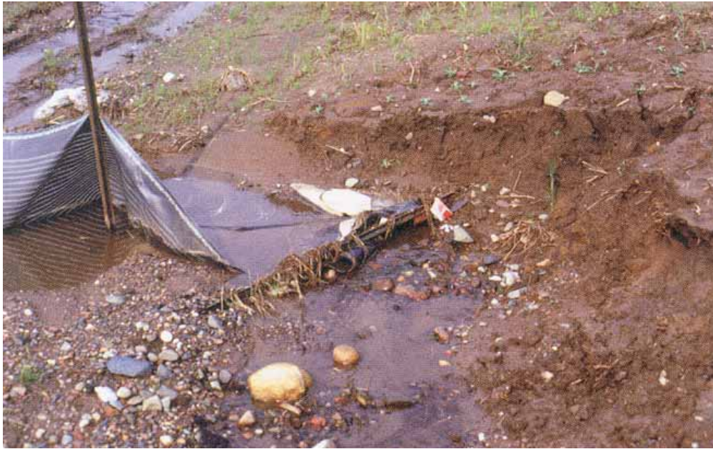
Figure 2.13. Improper silt fence installation (Source: Minnesota DOT)
