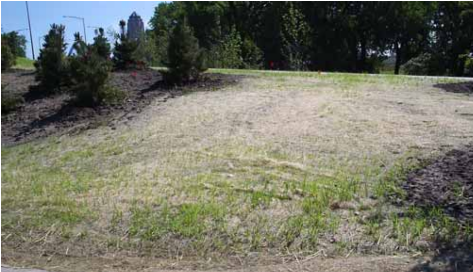
Figure 2.26. Foreslope protection in growth stage (Source: Department of Civil, Construction, and Environmental Engineering, Iowa State University)
