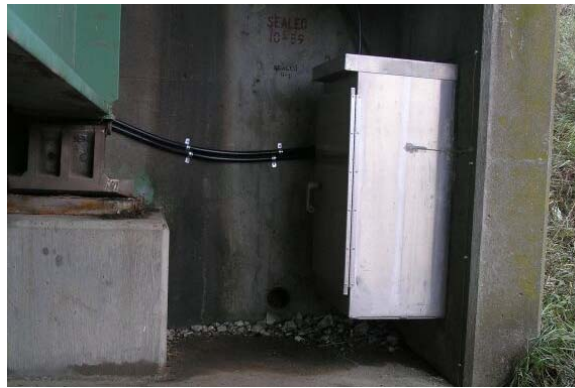
Figure 7. Aluminum cabinet mounted on the north corner of the west abutment wing wall
