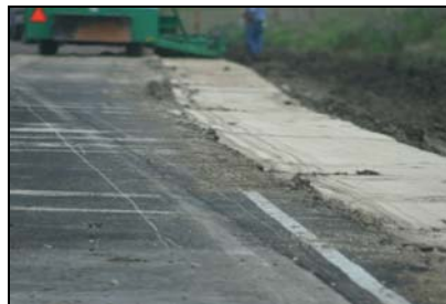
Figure 5. Edge line damage due to shoulder maintenance
