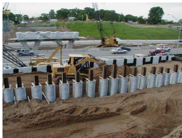
Figure 8. Piles in corrugated metal pipe sleeves for MLK Parkway bridge over I-235
