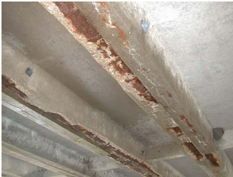
FIGURE 4. Typical PCB Deterioration
