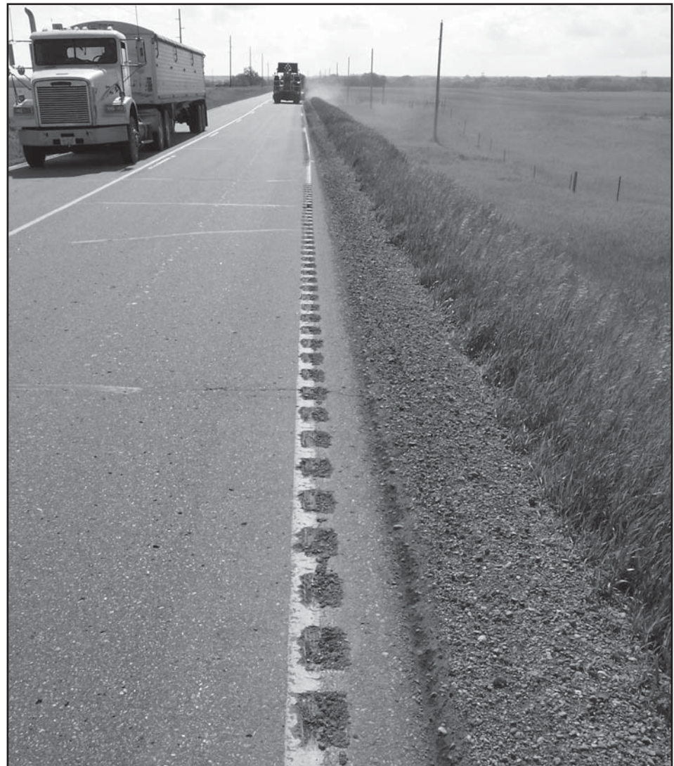
Milled-in rumble strips are applied to a county road, which will soon be painted over with edge line striping resulting in a "rumble stripe" (photo courtesy of Bob Sperry, Iowa LTAP).
